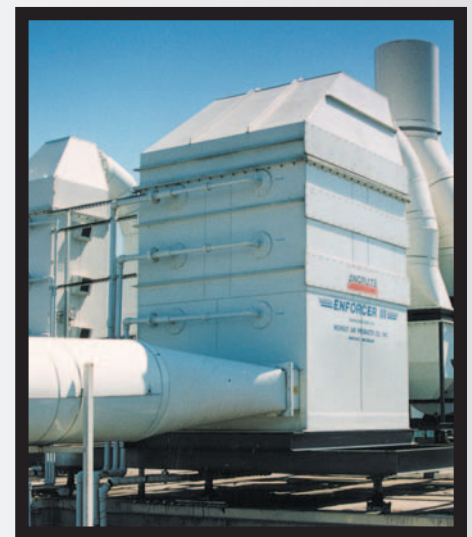
Tight control of production chemicals and careful management of air and water emissions are top priorities at Anoplate.
